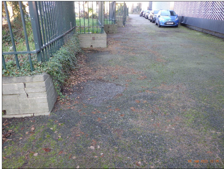
Figure 7 - Damage to car park
