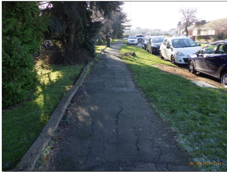
Figure 1 - Damage to footpath
