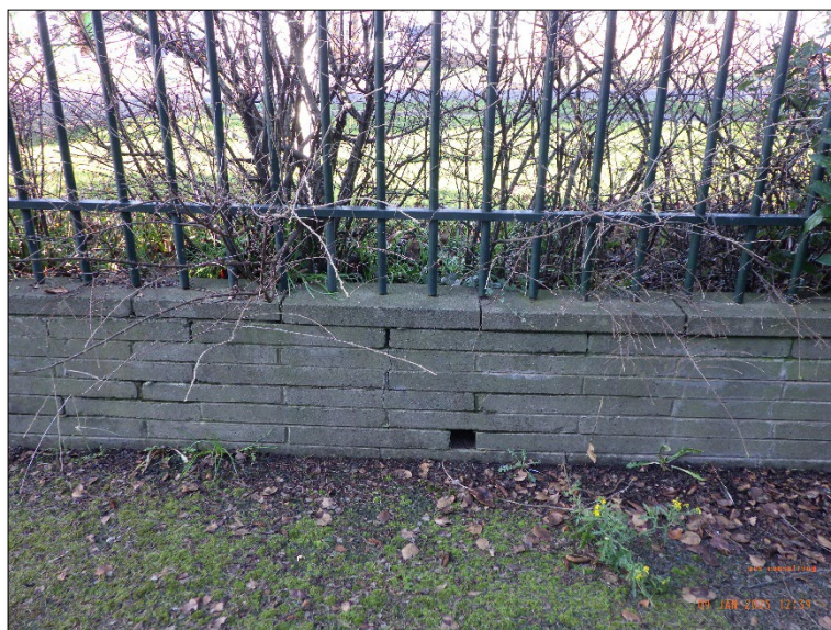
Figure 6 - Damage to retaining wall
