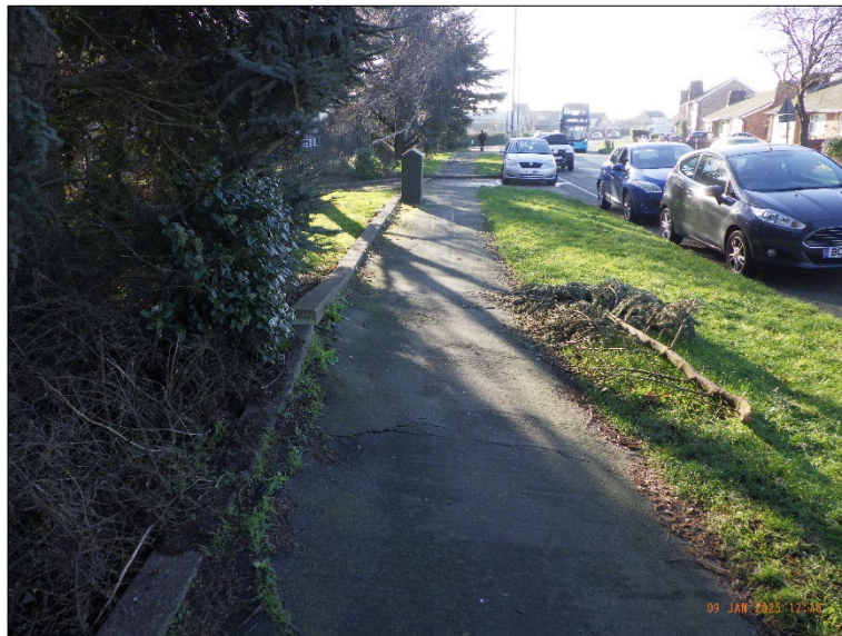
Figure 2 = Damage to footpath
